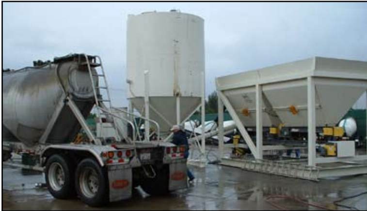
Filling Cement Silo
